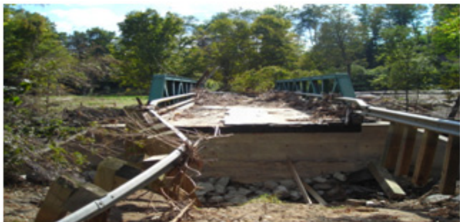
Major road damage in Roxbury, VT
