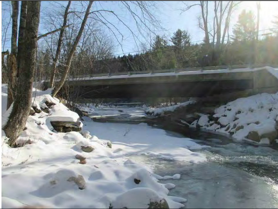
Mill Brook – Mill Brook Road (RT17) bridge No. 02- Entrance to bridge (RS 8966.95)
