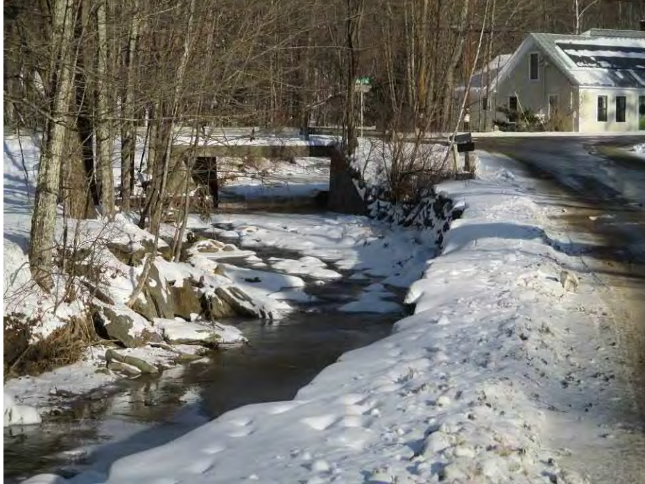
Freeman Brook – Outlet of the Brook Road bridge No. 01 in Warren Village (RS 1058.64)
