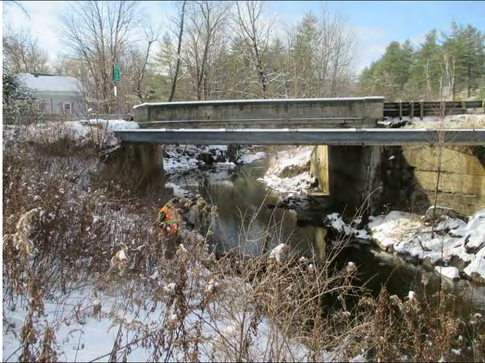
Thatcher Brook – Entrance to Stowe Rd bridge (sewer or water main in front of bridge) (RS 5970.35)
