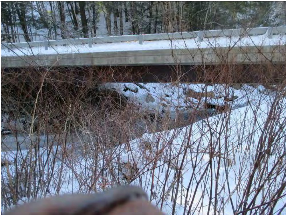
Mill Brook – Mill Brook Road (RT17) bridge No. 03- outlet of bridge (RS 11109.40)
