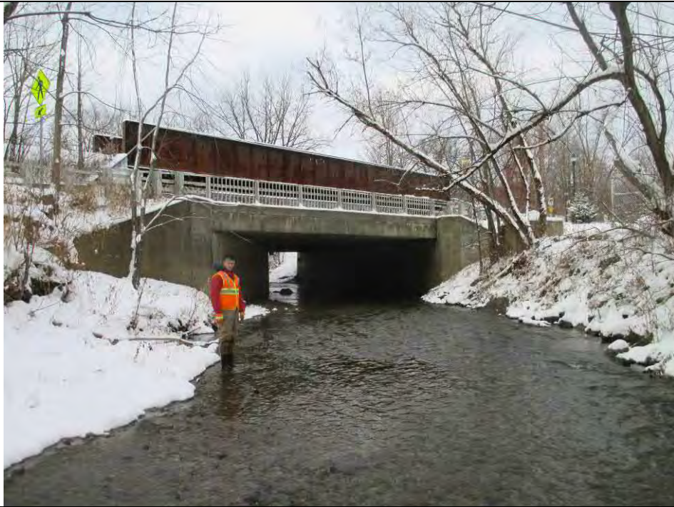
Thatcher Brook – RT 2 - N. Main- Union and Railroad bridge – Entrance to bridge (Union Street) RS 1051.27
