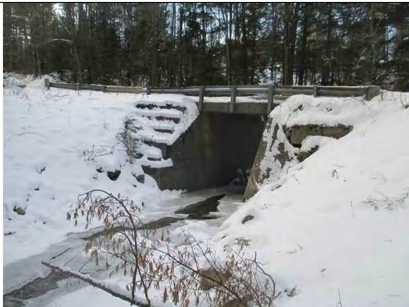
Freeman Brook – Entrance to a bridge on Behn Road in Warren (RS 9431.22)
