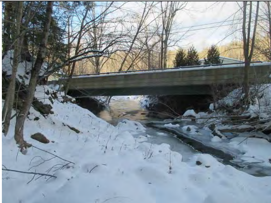
Freeman Brook – Entrance to Brook Road bridge No. 02 in Warren Village (RS 2068.04)
