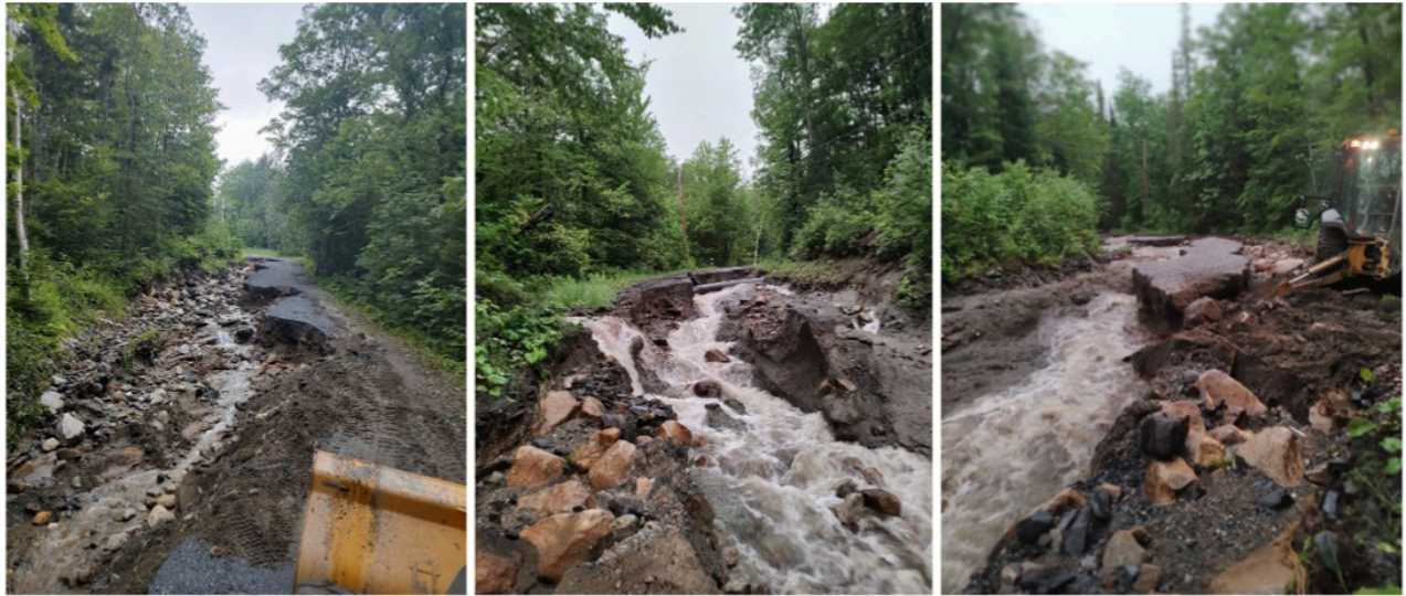
Provencher Road, July 2023 Flood Damage (Photo Credit: John Barnes)
