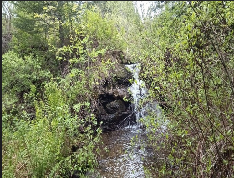
breached dam at pond outlet
