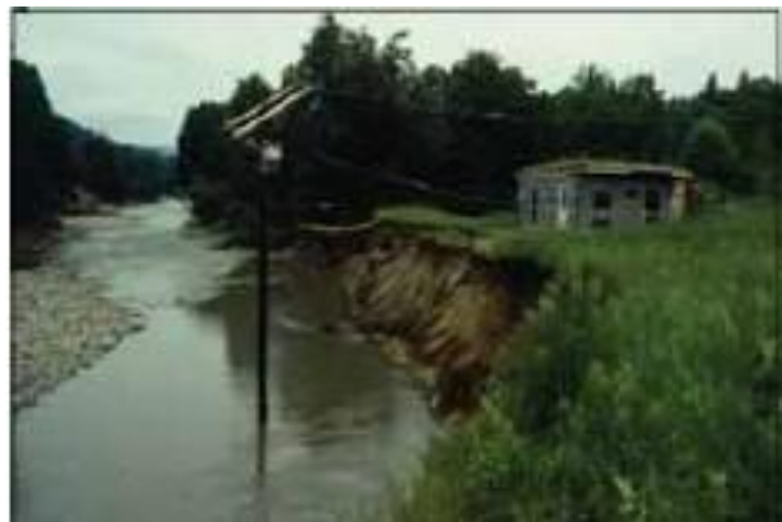
Fluvial erosion along the Mad River, Waitsfield, Vermont. Image courtesy of VTDEC River Management Program.
