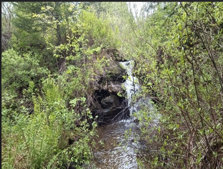
breached dam at pond outlet
